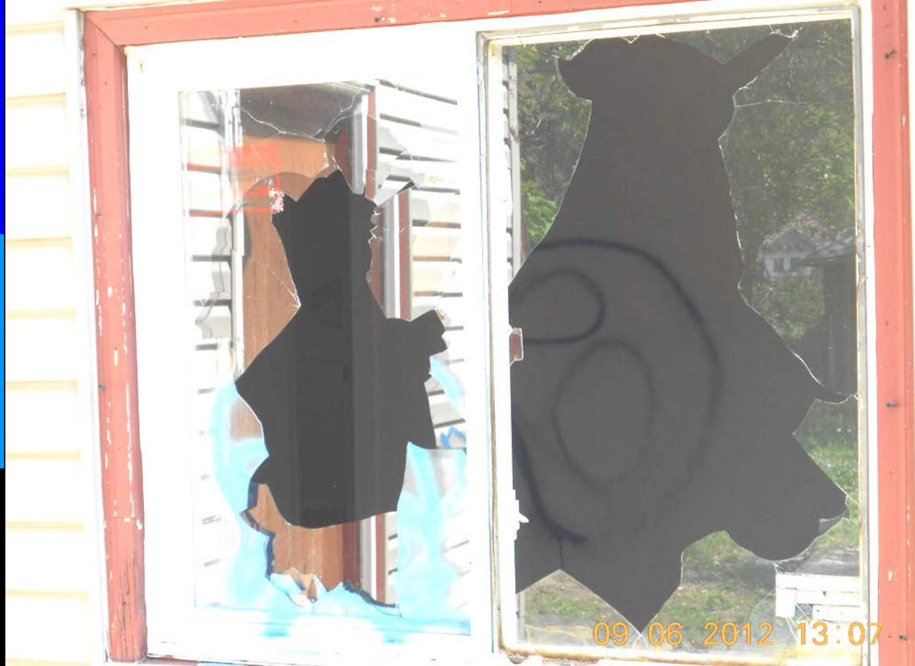
You can also see graffiti inside the home through the broken windows.
