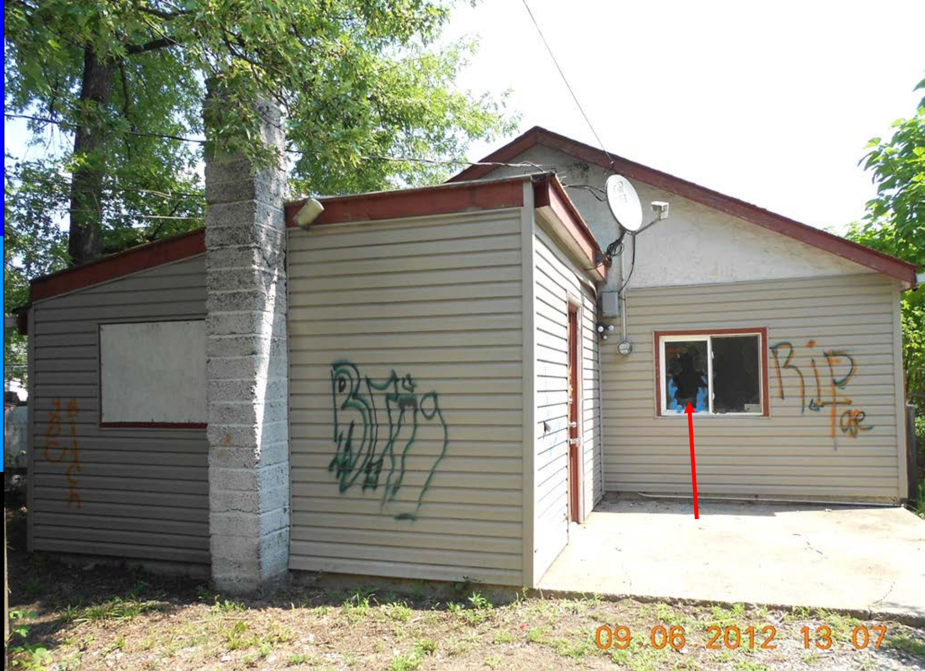
Fannie Mae's neglect invited vandalism and graffiti to this home – note the broken window as well.
